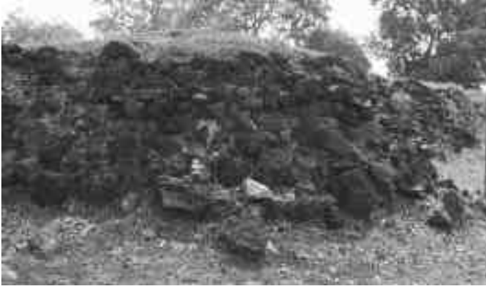
The crumbling bastion as you enter.
