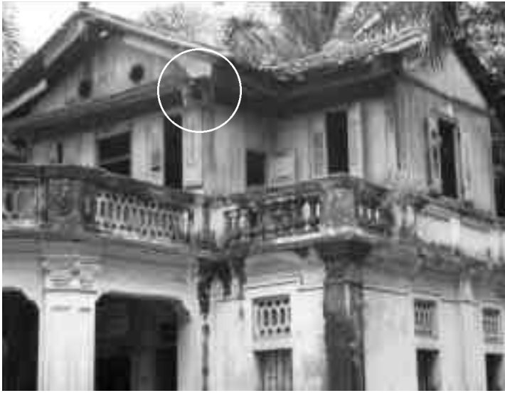
Timber roof bracket usually found in Chinese temple construction rather than in domestic architecture.
